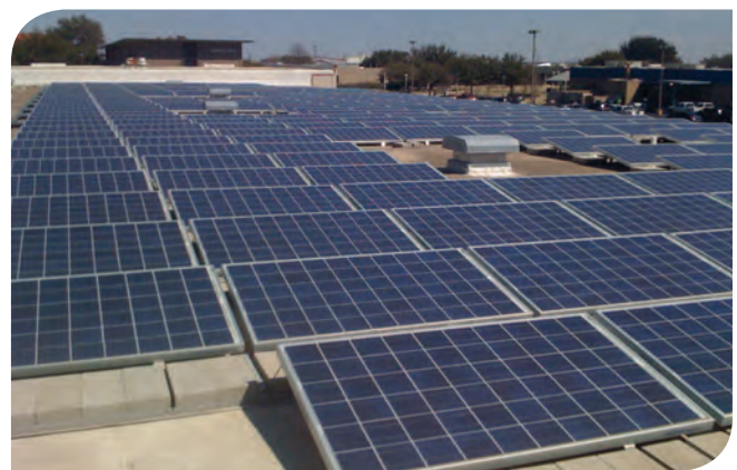
Renewable energy was included in the upgrade, with a 100 kW solar PV system and a new roof installed on one of TSTC's classroom buildings.
