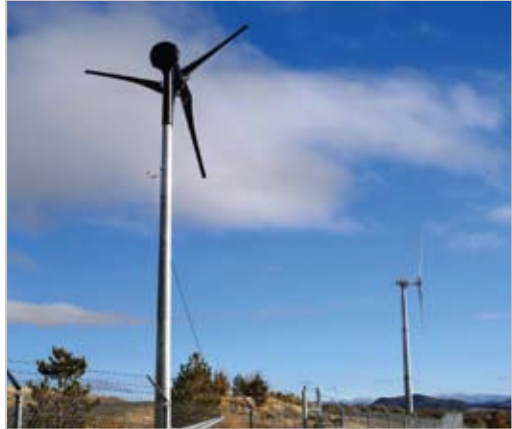
Ameresco installed two wind turbines at the City of Reno Stead Waste Water Treatment Plant.
