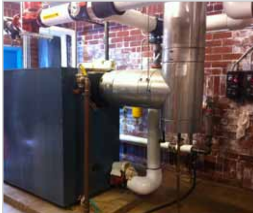
Above is one of the boilers inside the boiler room at the Captain Strong Primary School. The partnership with Ameresco under an ESFC will enable the District to upgrade old equipment and become more efficient without imposing constraints on local taxpayers.
